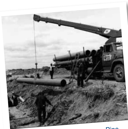
450 mm (18") PVC Pressure Pipe in service for 27 years in Varennes, PQ
