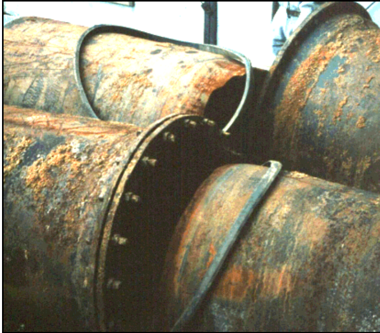
Photo 5. Ductile iron pipe joints that telescoped when they were put in compression. Kobe 1995.
