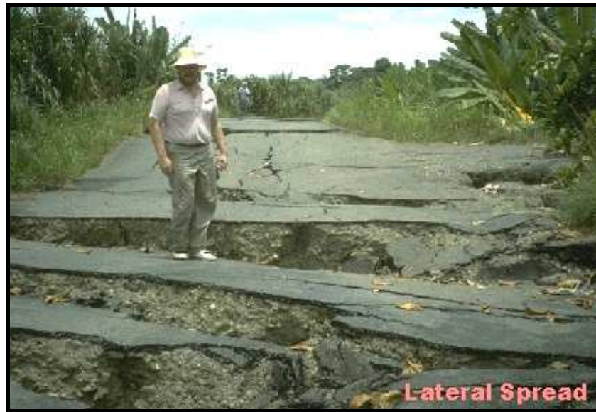
Photo 3. Liquefaction induced lateral spreading (Costa Rica 1991)
