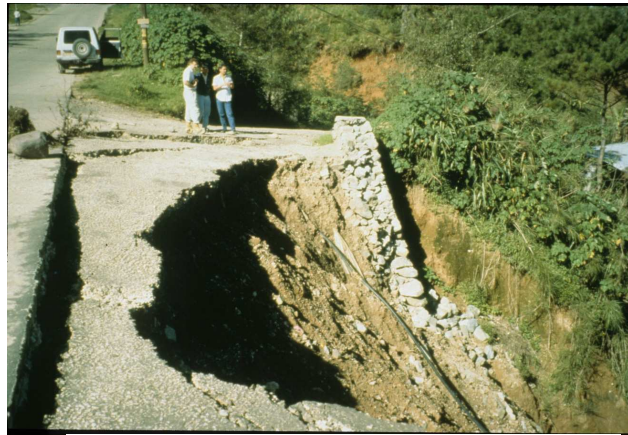
Photo 4. Landslide beside a road fill area (Philippines, 1990)
