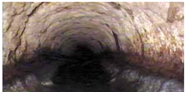
Sulfuric acid causes severe damages to concrete pipes and manholes over time.
